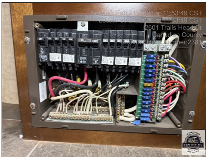
Power Distribution Panel
