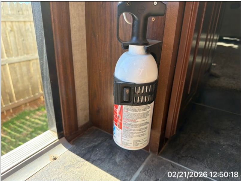
5-B:C Fire Extinguisher
