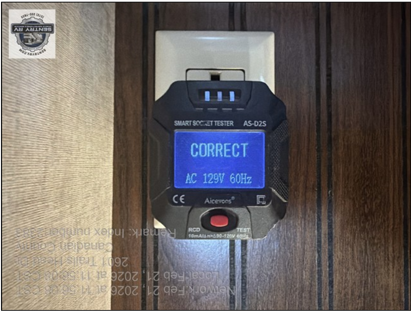
Voltage/Polarity/Frequency Test Rear Wall
