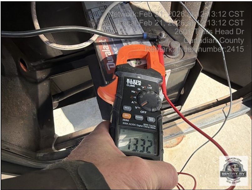
Battery Voltage Shore Power ON
