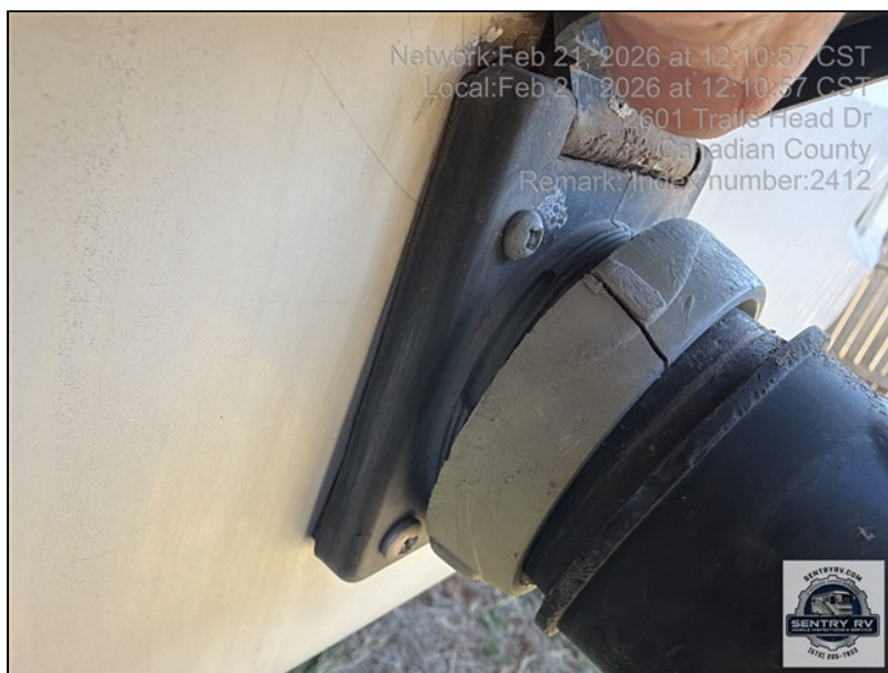
Cracked 50 Amp Retaining Ring
