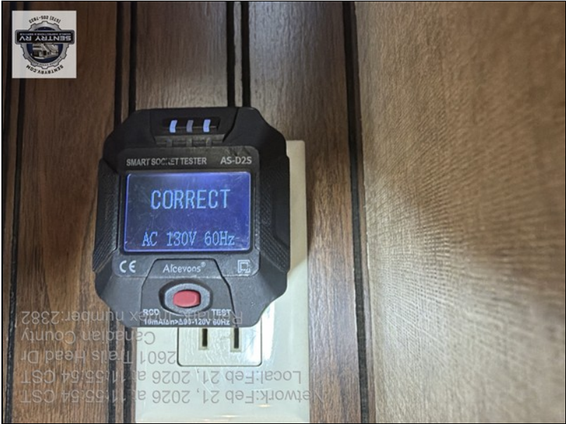
Voltage/Polarity/Frequency Test Rear Wall
