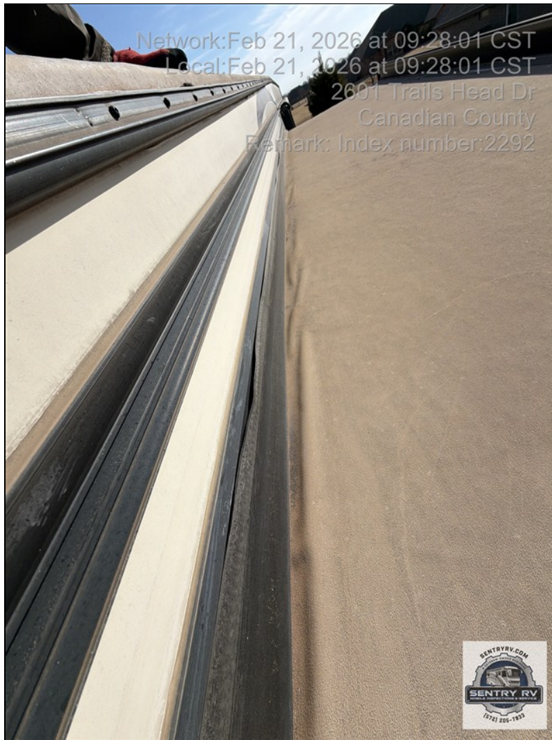
Curbside Slideout Seals
