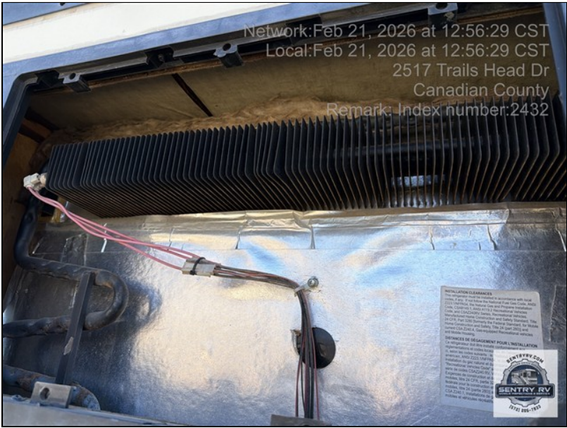
Incorrect Upper Ventilation
