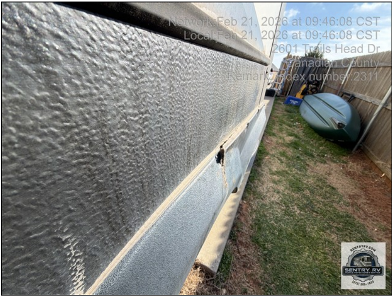
Wheel Well Crack
