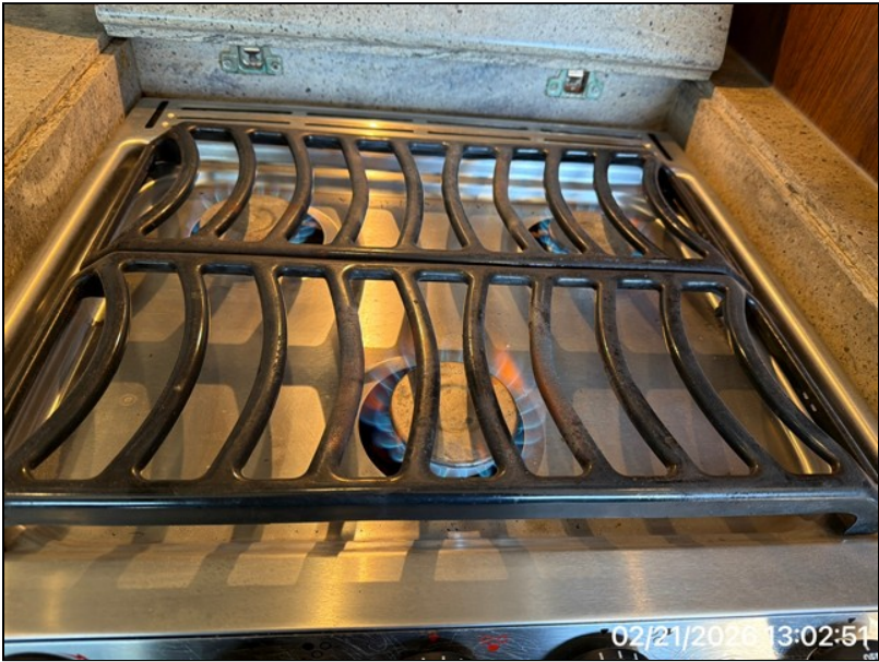
Cook Top Burner
