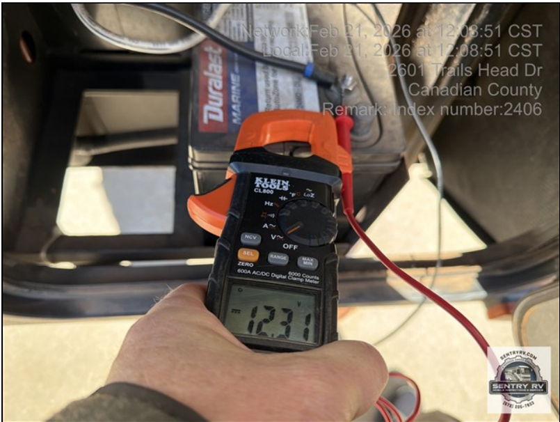
Battery Voltage Shore Power OFF
