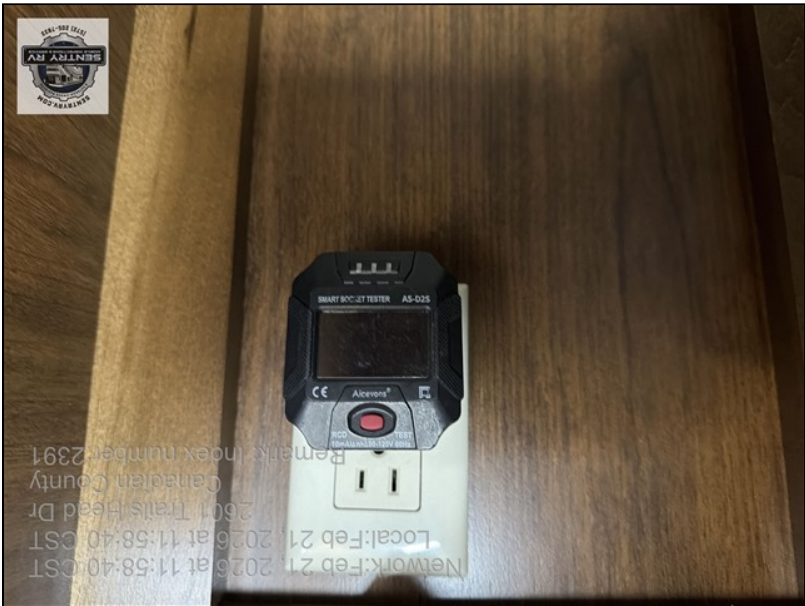
No Power in Closet Outlet
