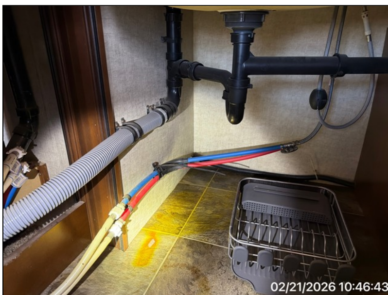
Stain Under Kitchen Sink
