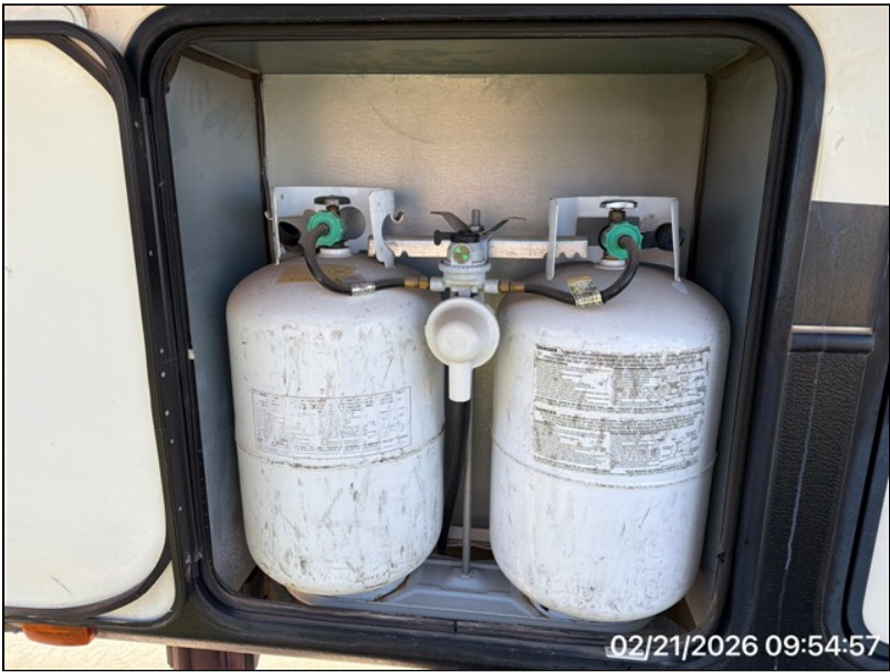
Streetside LP Storage
